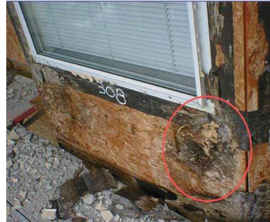
Window water leakage will cause damage to wood framing regardless of differences in drying potential
