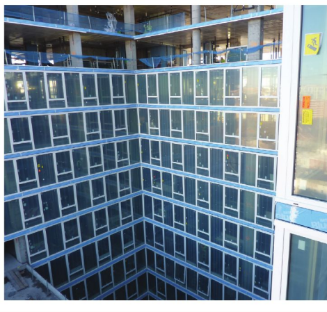
View of window products installed in a window wall application between slabs. However, exterior access is still required to complete the exterior perimeter seals and install the slab edge covers.
